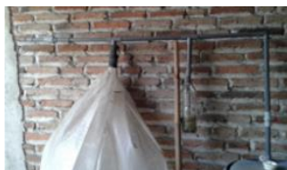
c. Reservoir Biogas
